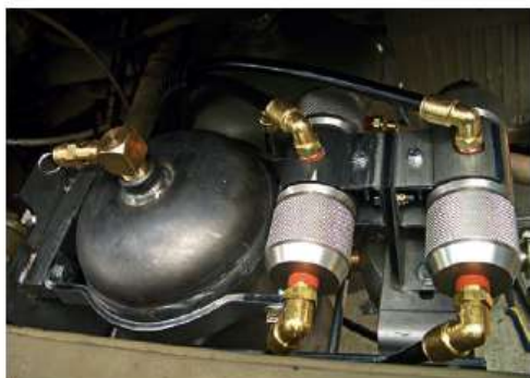
DOT fittings in service.
